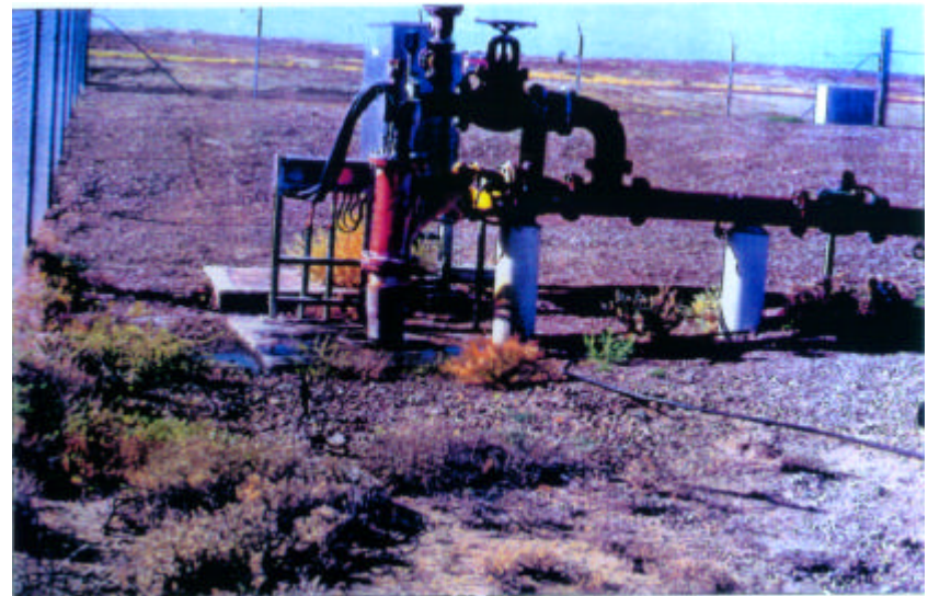
Figure 24 - WMC Bore, Lake Eyre South
